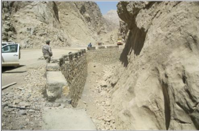
Above: The road project linking Parwan and Bamiyan Provinces is a seven-phase process with hopes of improving economical stability
